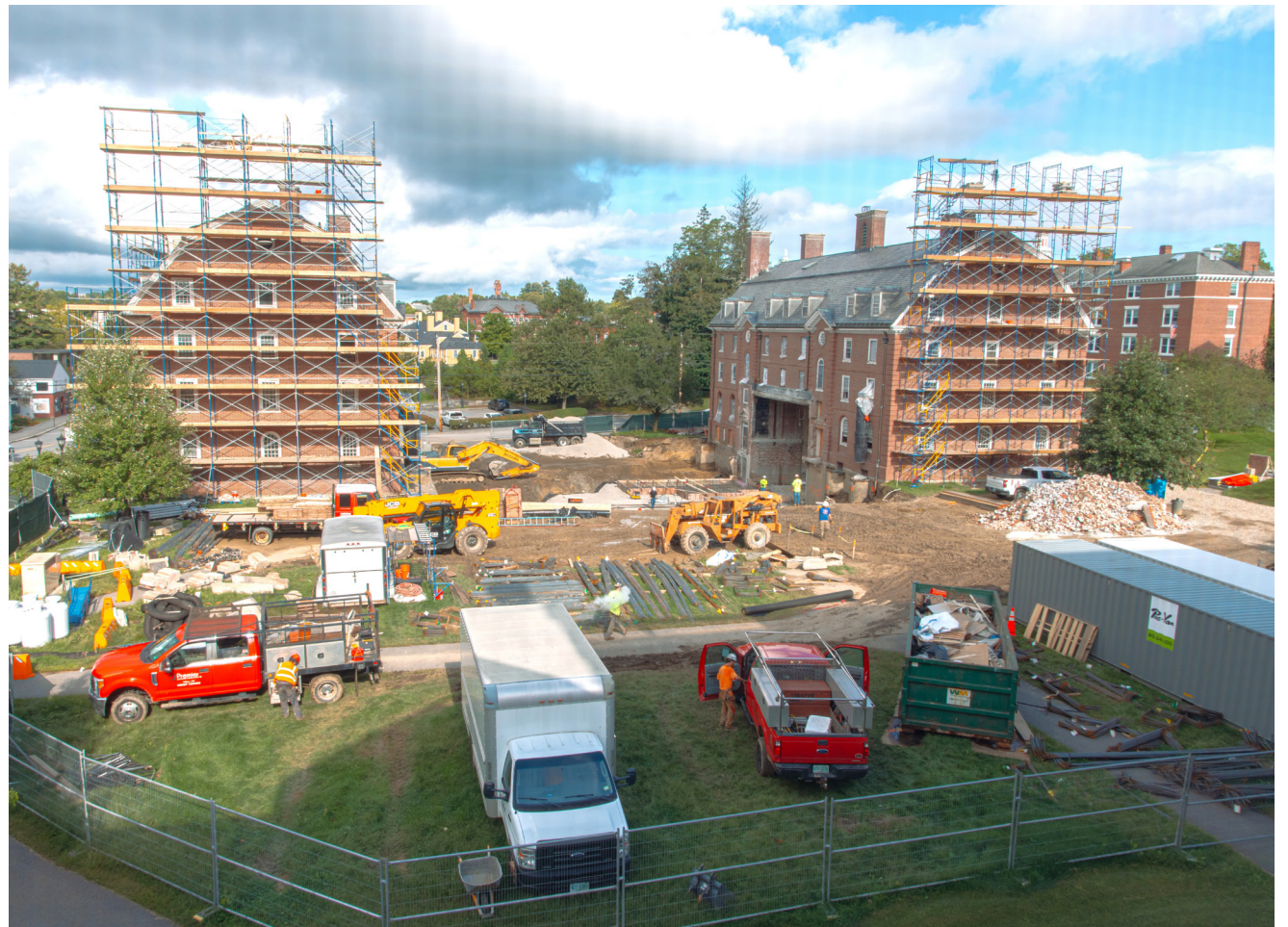
Exeter construction includes rebuilding a new dining hall and renovating Merrill and Langdell Halls.
